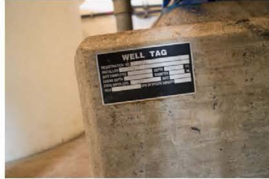
Photo 54 – Public water well tag (off of Aiken Ave)
