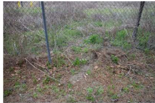
Photo 22 – Hole under fence on southern side of property
