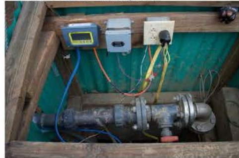
Photo 12 – Pump and treat system shed
