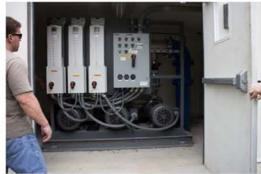
Photo 56 – New pumps/backup generators off of Aiken Ave
