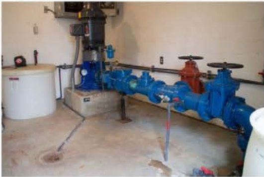
Photo 55 – Public well off of Aiken Ave
