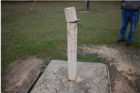
Photo 15 – Out of service monitoring well
