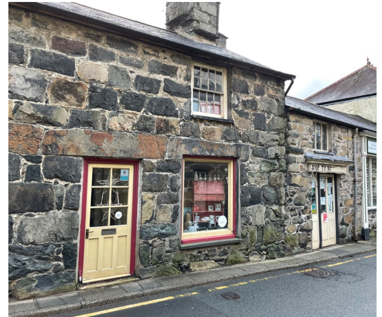
46 Roughly coursed stone, often dolerite, note the small stones between the large blocks almost 'galletting'. (2021).
