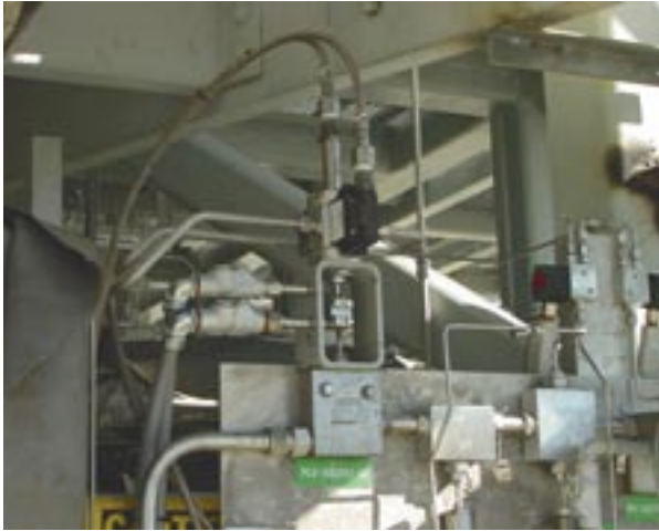
The high-pressure gaseous oxygen panel which feeds the ignition system for a rocket engine combustion device, located at ground level on the E-I Test Facility, Cell 3. The valve identified as PCV-10A2892-GO is operated by means of the high-performance actuator developed as a part of the Dual-Use Cooperative Agreement with BAFCO, Inc.
