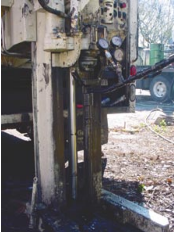
Weston Solutions, Inc.'s Emulsified Zero-Valent Iron remediation technology in process at a client site.
