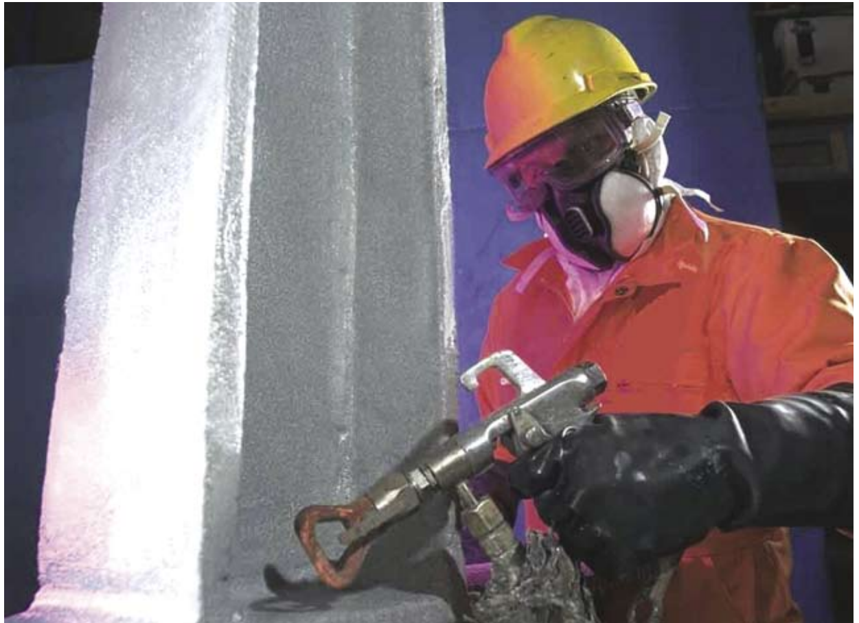
Fabrication shop application of Interchar fireproofing material to structural steel beams. Since Interchar is typically applied at a thickness between 1 and 8 millimeters, it does not impact the overall shape of the steel. This means architects and building planners can still explore intricate and innovate architectural designs.
