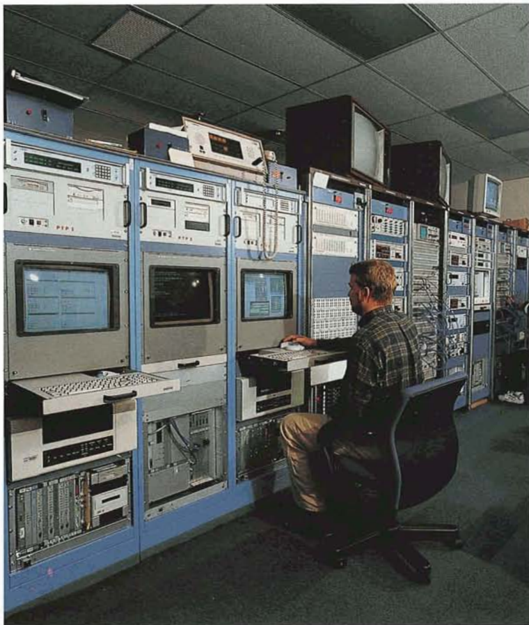
Avtec has provided telemetry hardware in support of NASA’s Communications Network (NASCOM). Shown are NASCOM boards at Goddard Space Flight Center’s Simulations Operations Center.
