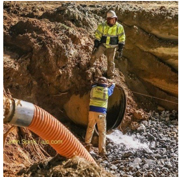
2018 Atlanta Water Main Break
