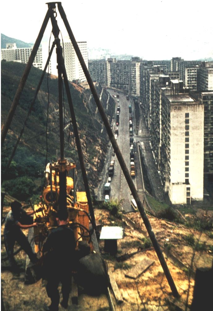
Figure 11: Drilling vertical diamond core holes into the Sau Mau Ping slope. These holes were used for geotechnical investigation purposes and for the installation of piezometers in the rock mass.
