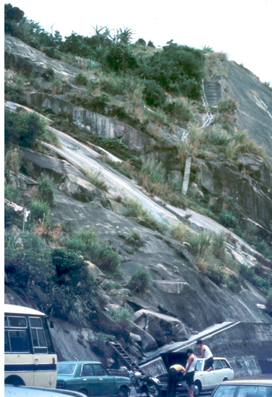
Figure 4: The failure surface defined by a sheet joint surface on which a small slide occurred during blasting of the original cut slope for the Sau Mau Ping Road. The potentially unstable slope discussed is visible in the background.
