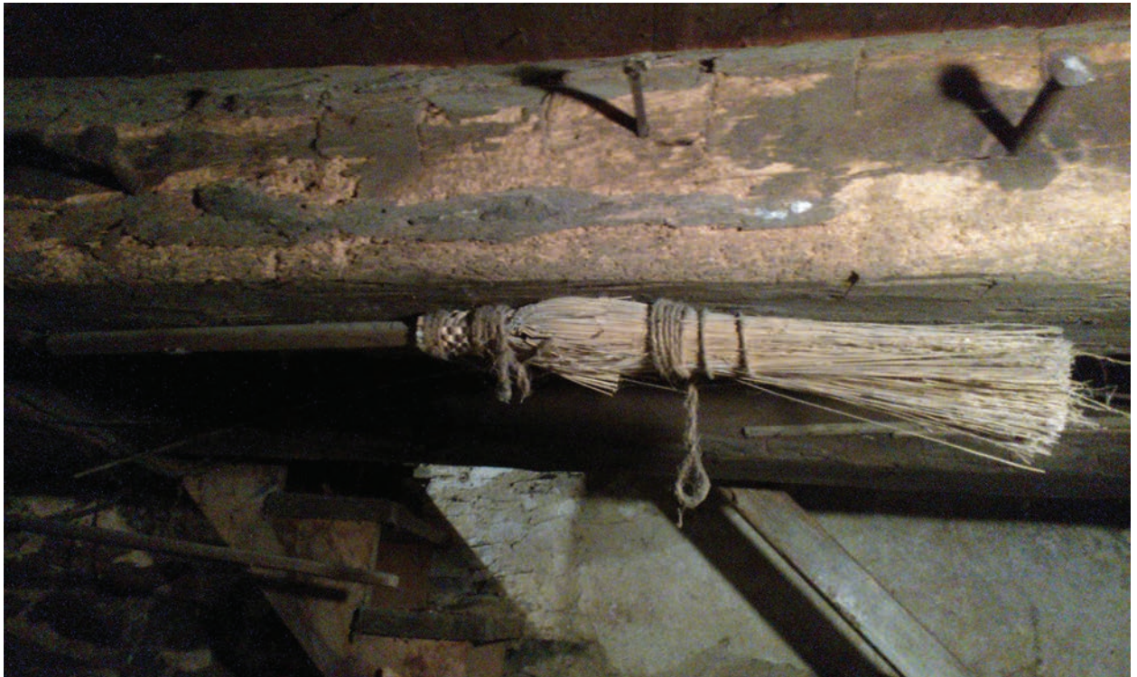
A concealed broom in a Berks County farm house, nailed to a floor joist visible by the basement stairs. Private Collection.
