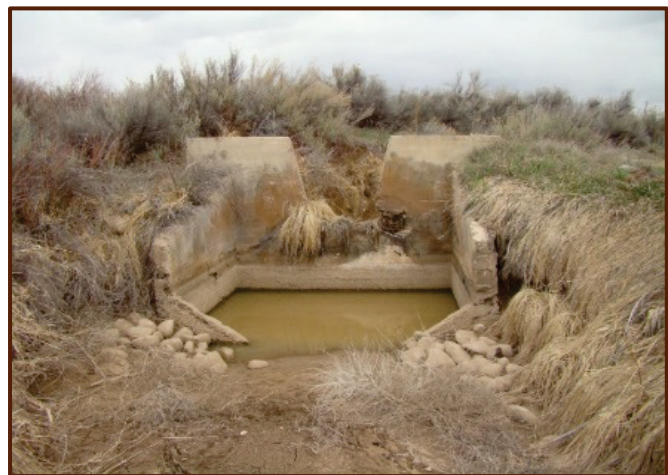
Significantly deteriorated infrastructure hampers irrigation water delivery to portions of the Southern Ute Reservation. Photo courtesy of Southern Ute Indian Tribe
