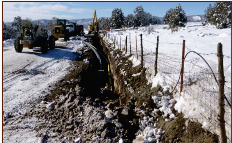
Rural domestic water systems can require miles of pipeline to serve only a small number of residences, increasing the per user costs for both construction and maintenance.
