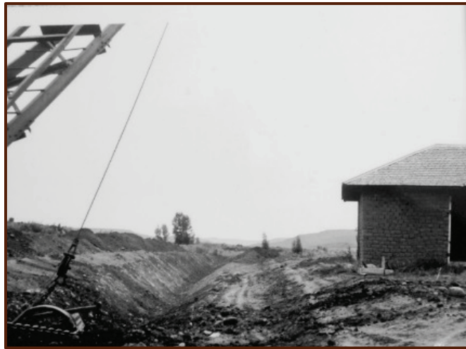
Rehabilitation of a Tribal canal in the Pine River valley using a dragline – circa 1964.
