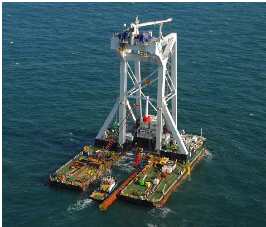
Figure 8. The piling vessel Svanen, with a monopile ready to be lifted and piled and the red and white hammer central in the image (Photo RBINS).
