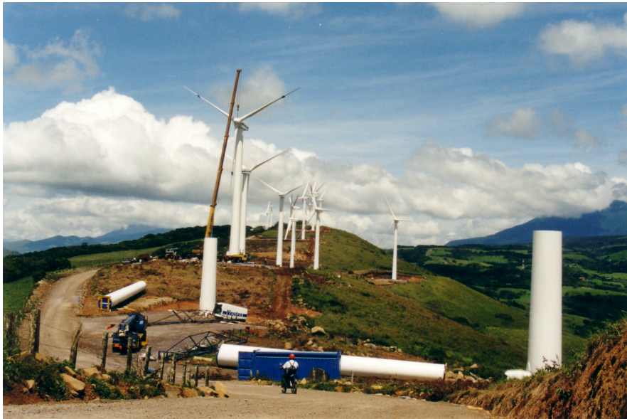
Fig. 12 The 20 MW wind farm on Montecristo during construction works. The impact due to excavations for foundations and cable trenches can be clearly visible. The revegetation will cover these scars quite soon however, turning it green again.
