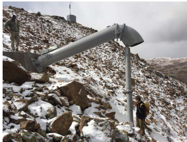
Figure 25. 1.5 m 3 Gazex installation at Loveland Pass, Colorado. Photo: A.Jones.
