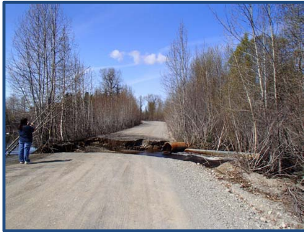
Road washout as a result of an undersized culvert on Indian Creek in May, 2012.
