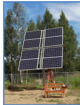
Solar array at Tyonek community garden, installed 2013
