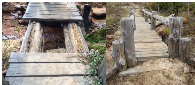
Bridge at Bastrop State Park. Damage from Hurricane Harvey (left), and after Bridge Maniacs repairs (right)
