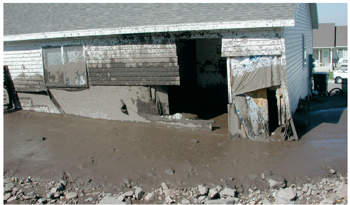
The debris flow broke through the back wall of this house on Peach Street in Santaquin.
