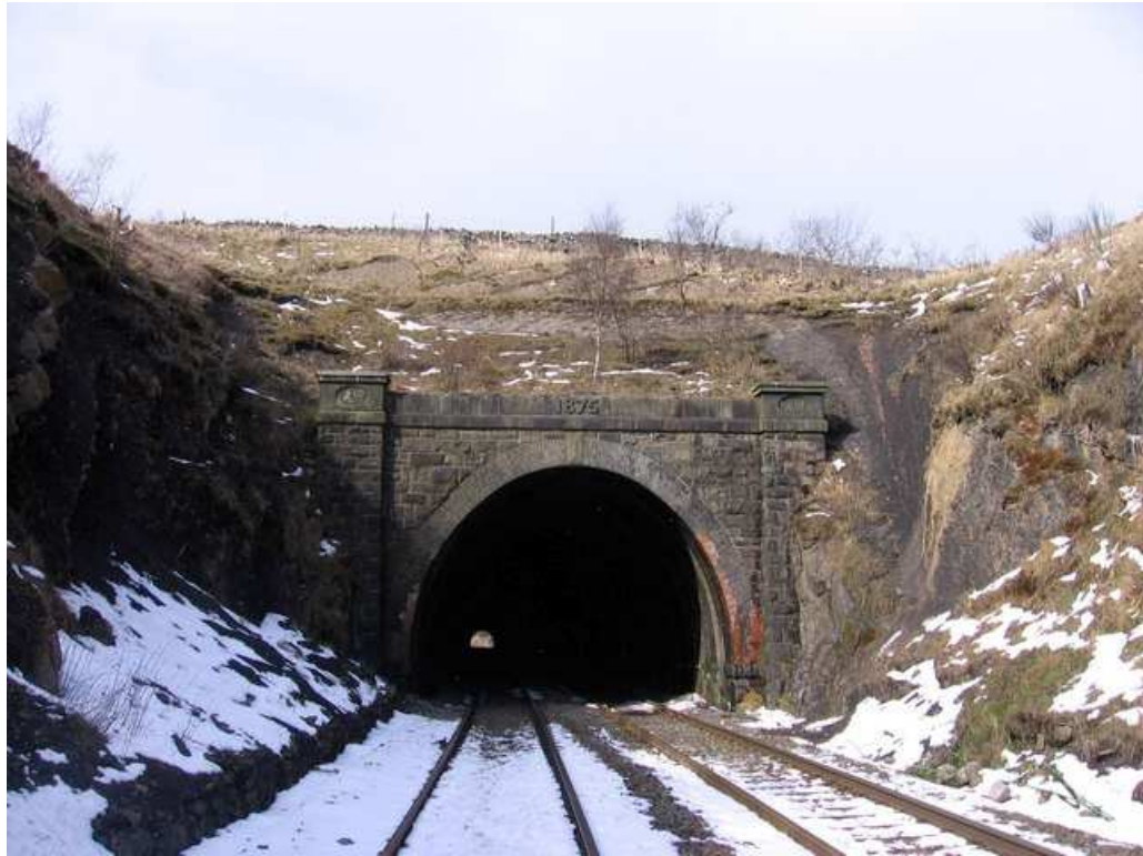
Plate 10: A view of the southern portal of Birkett Tunnel (Site 04 ) of the Settle and Carlisle Railway
