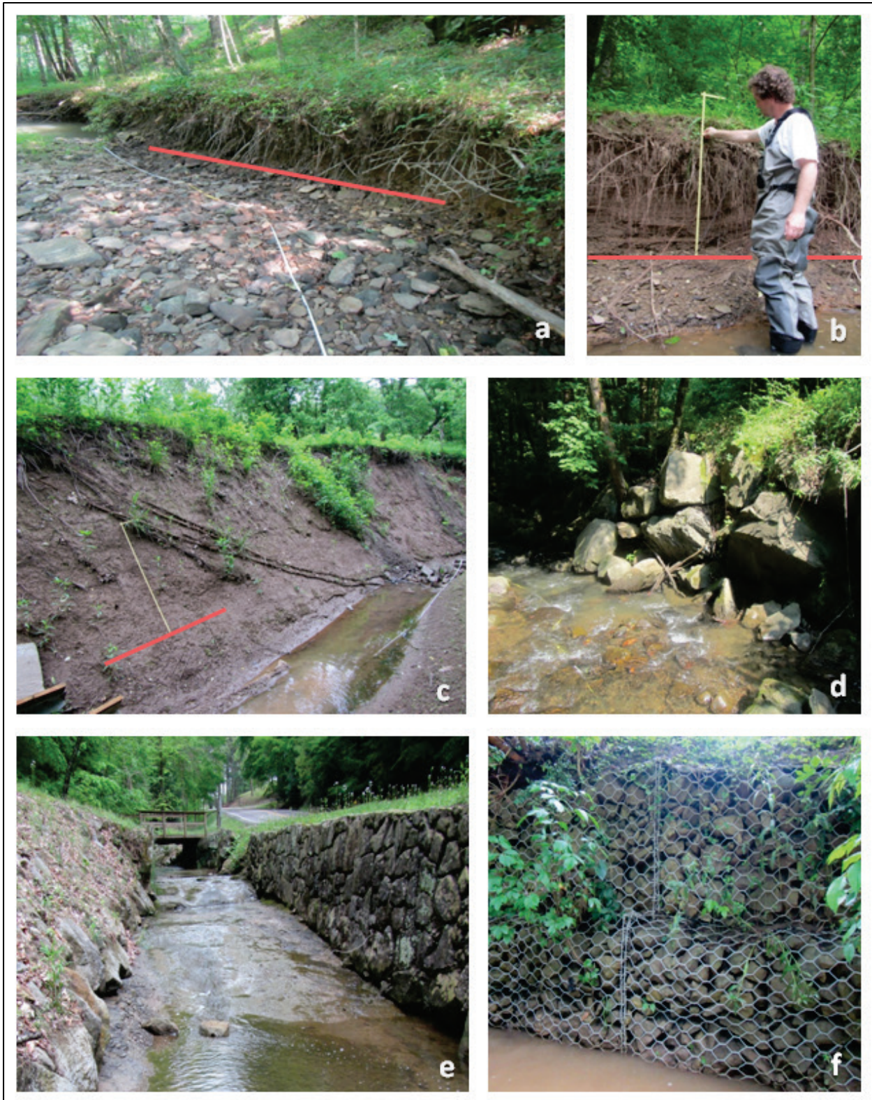
Figure 20. Examples of erosion height categories (bankfull stage indicated by red lines): (a) erosion 0.1–2 ft above bankfull stage; (b) erosion 2.1–4 ft above bankfull stage; (c) erosion >4 ft above bankfull stage; artificial bank stabilization with (d) boulders, (e) concrete and boulders, and (f) riprap.
