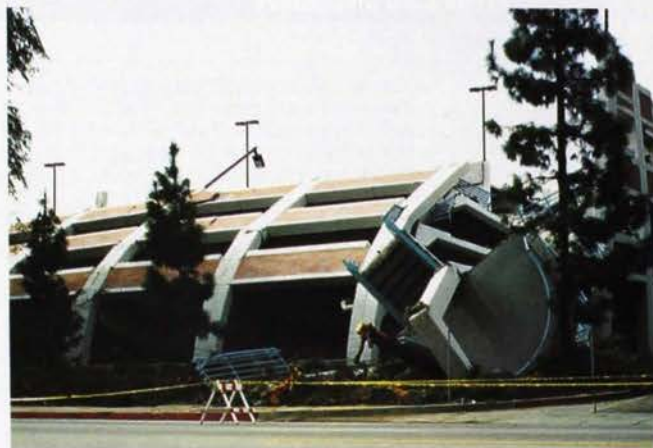
A university parking structure was one of the many damaged buildings at California State University, Northridge.
