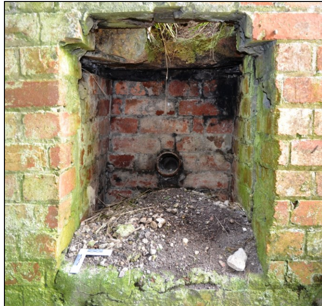
Fig. 8 Fire place in the blast shelter showing air in-let pipe and boiler plate
