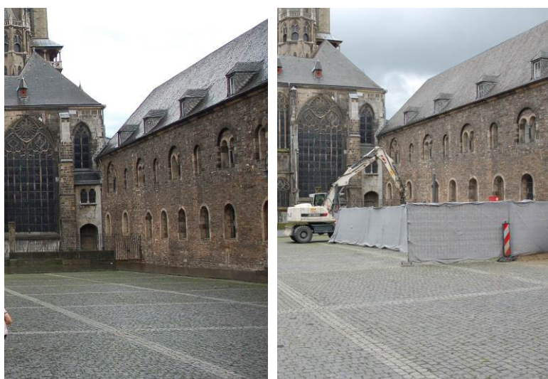
Figure 7 – Measurement location 6 with soundwalk participant in 2011 (left) and the same measurement location in 2012 (right). The construction machinery on the right picture was operating during soundwalk.
