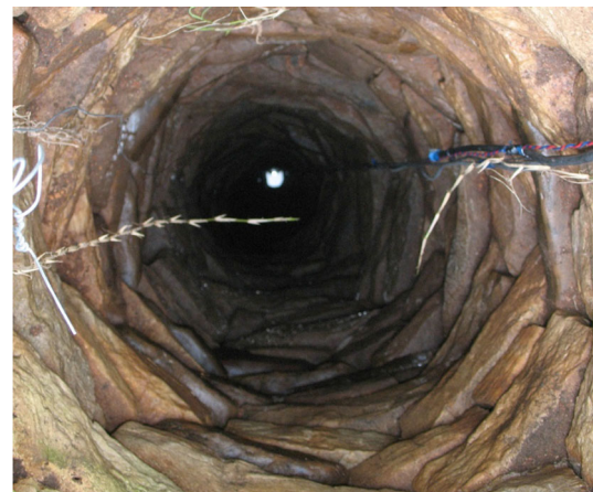
Fig. 8 View looking down well BS-36, which shows the groundwater reflected as a bright spot of light at a depth of 10.15 m below the top of the well. Cables and wires allow data to be communicated from below the water surface to the data recorder (Fig. 7). Hand-dug wells are not uncommon in the Big Creek area, and provide a glimpse into a bygone era when they were created by pick and shovel as the well digger was lowered by rope and pulley down to a level where he encountered water. Dug wells have to be wide enough to allow the well digger to fit inside the borehole, and this one is 0.46 m in diameter. When the well digger has reached the level where water moves into the well to a depth that hopefully does not dry up during droughts, his digging is completed. The walls of the borehole are often lined with sandstone or chert rock slabs that keep soil and other debris from falling into the well. Dug wells are an excellent means for hydrogeologists to gain direct measurement into the water that is flowing underground
