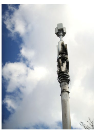
A telecom tower damaged by fire this month in Birmingham, England. Carl Recine/Reuters
