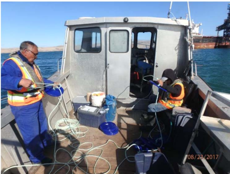
Photograph 26: Field team constructing settlement plates for deployment at Milne Port ore dock, 23 August 2017.
