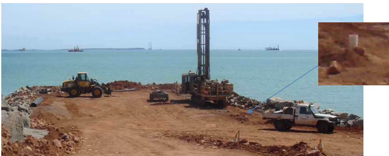
Figure 4 - The above image shows a drill rig working through a rock-fill platform constructed over a near-shore area. The insert shows a hole lined with a pvc pipe. The rig shown in the image is much larger than required at Rothera.
