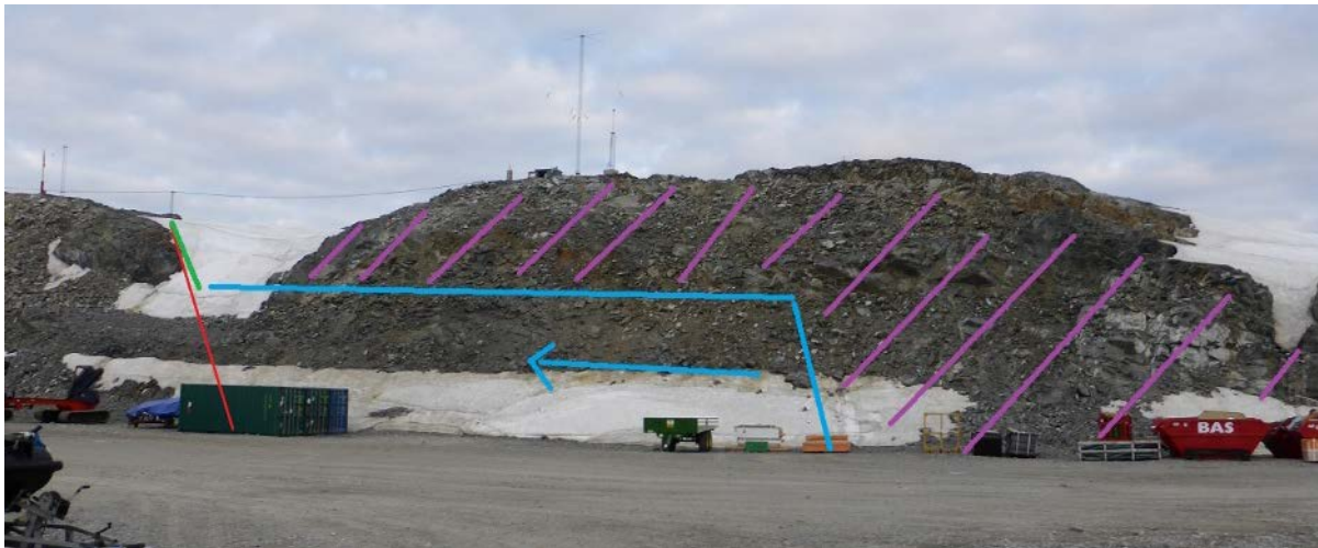
Figure 8 – Quarry stage 3 showing the upper bench worked out and production continuing on the lower bench.
