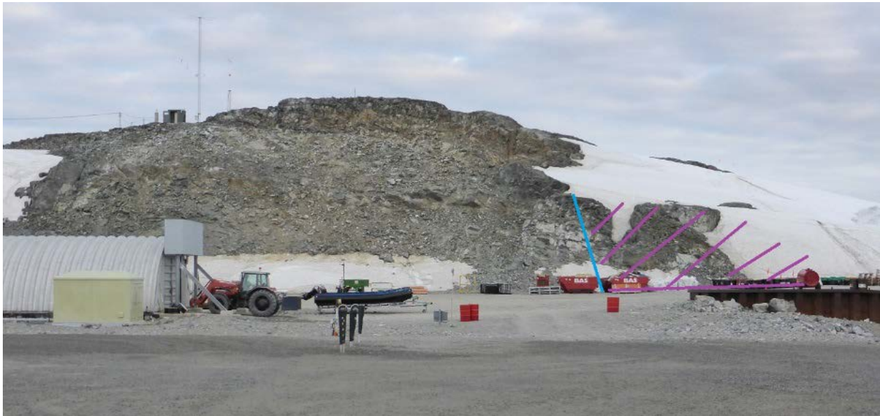
Figure 4 – Quarry stage one image from the west, showing the rock to be removed in purple hatching.
