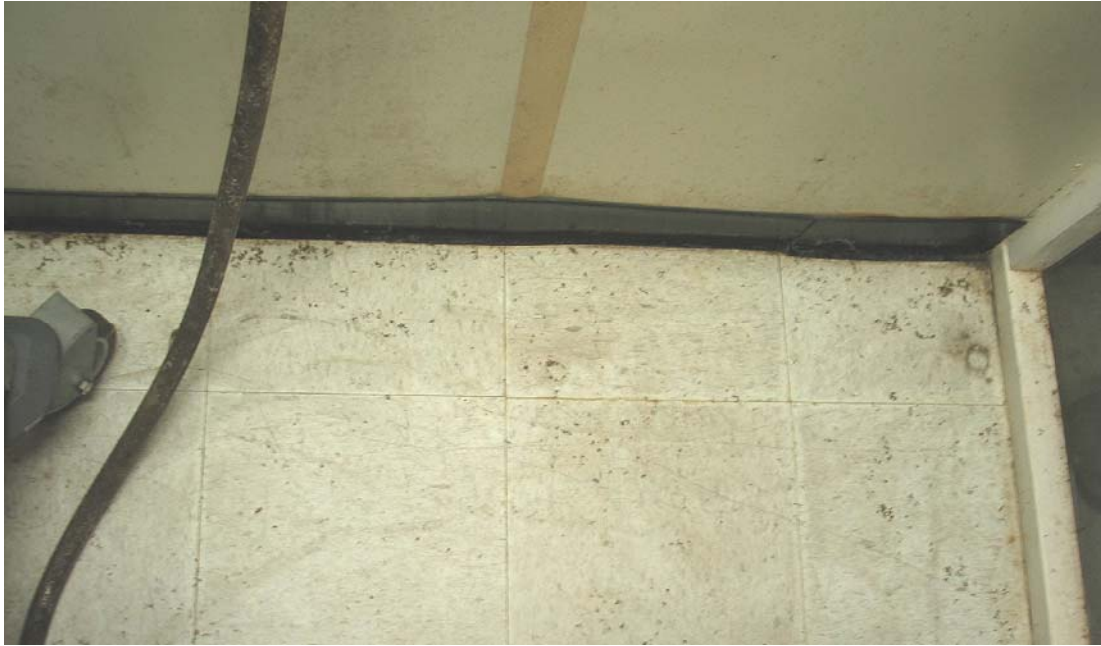
Figure 1.2.7. The mildew and mold growth on the walls and the floor of this insectary can stress mosquitoes causing them to be more susceptible to infections and less able to respond to changing conditions.
