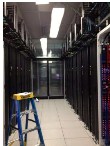
Figure 7: Typical server rack “contained” warm aisle
