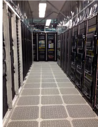
Figure 6: Typical server rack cold aisle
