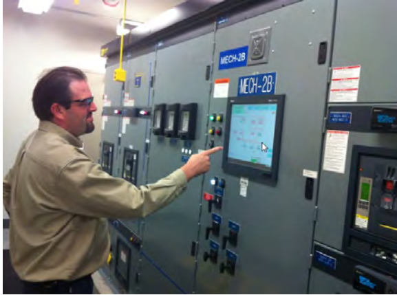
Figure 15: ACFM monitoring electrical gear
