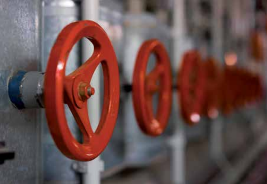
The heating supply under the public greenhouses
