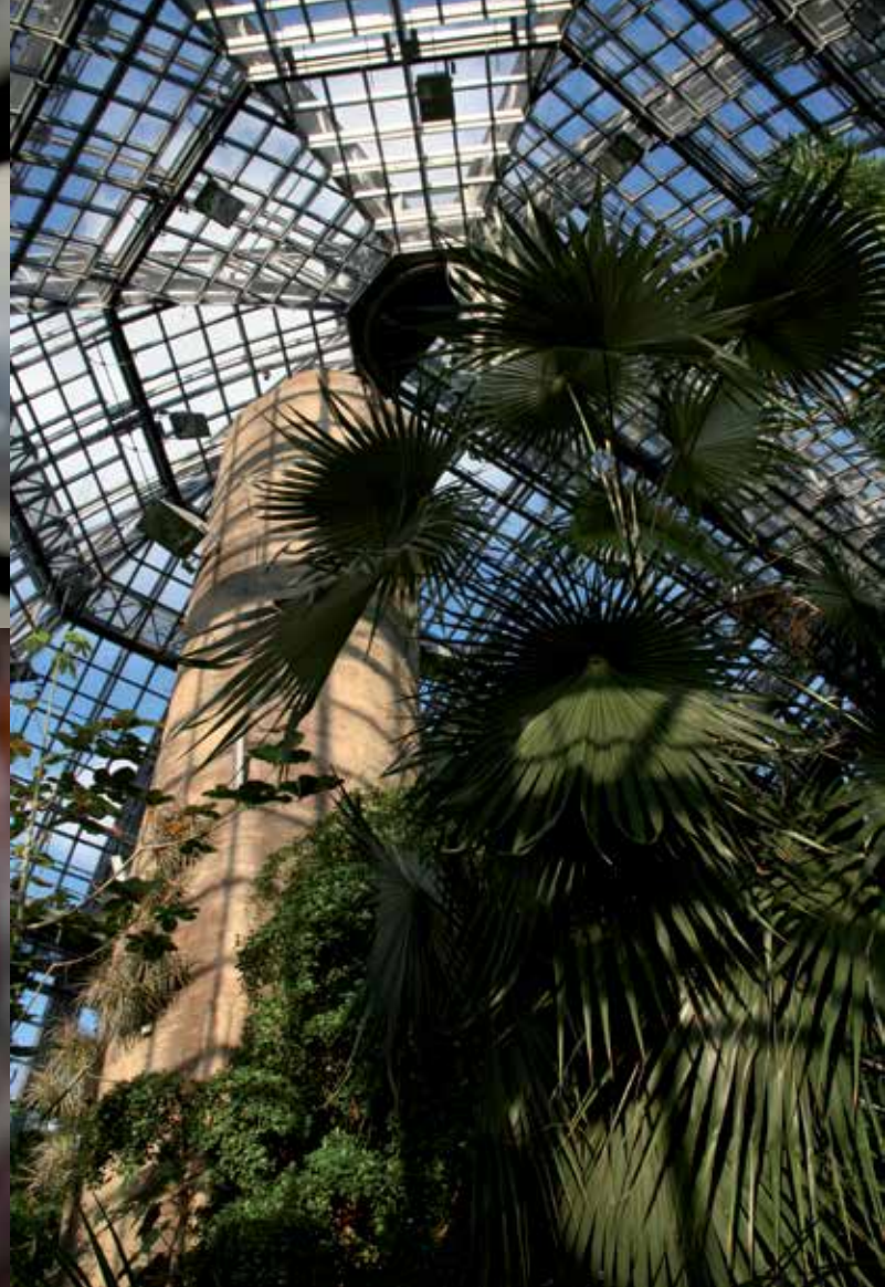
Towers camouflaged as tree trunks ensure that warm air is distributed through the Main Tropical Greenhouse
