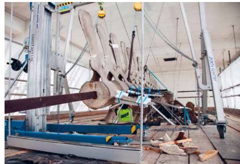
Figure 5. A large gantry was used to support the main armature while vertebrae were removed and cables were uncoupled.
