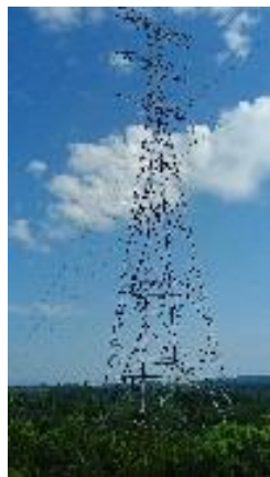
Photo 5: Transmission line "Río Frío" farm.
