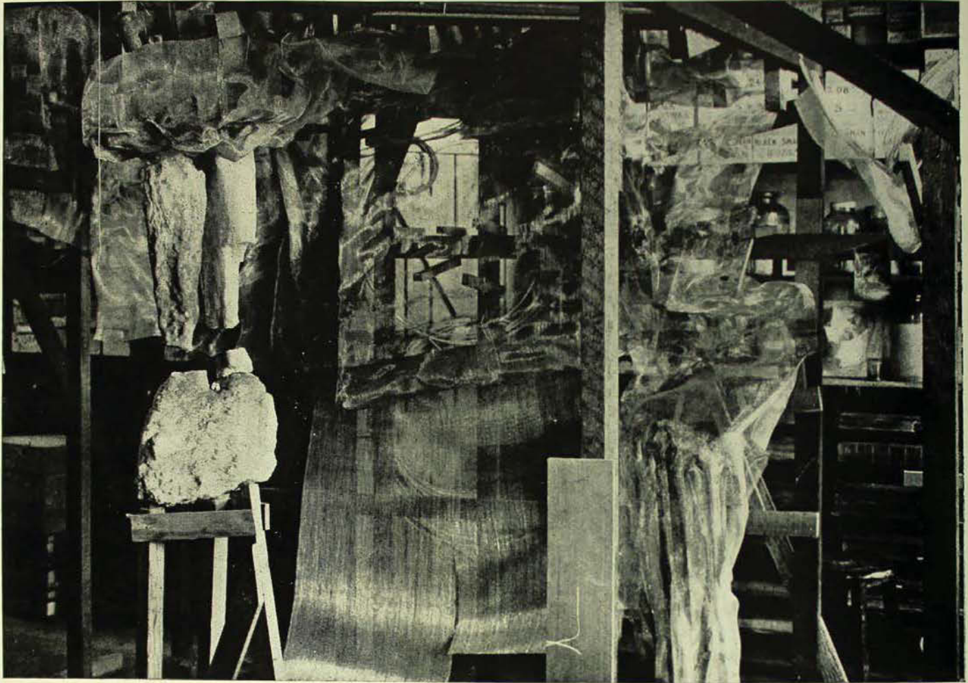
A start is made with the construction of the Cave Group. The broken column is placed in position, and the laying of eight hundred square feet of wire gauze is commenced on the outer framework.
