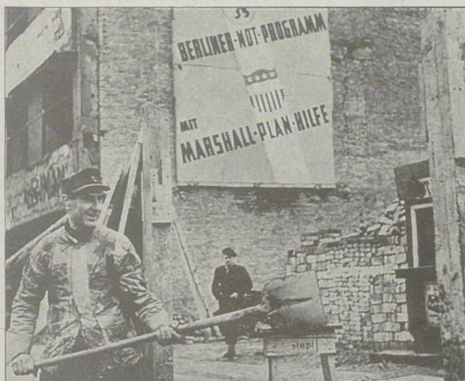
This worker became a symbol of Berlin's recovery (1950), as he prepared to lay the foundation for a Marshall Plan, low-cost housing project.
