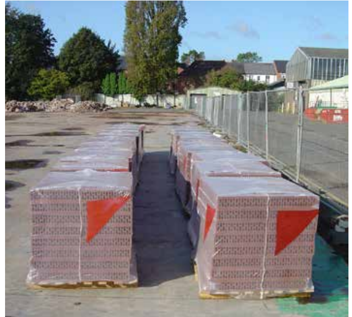
Good storage with recycled plastic cover.
