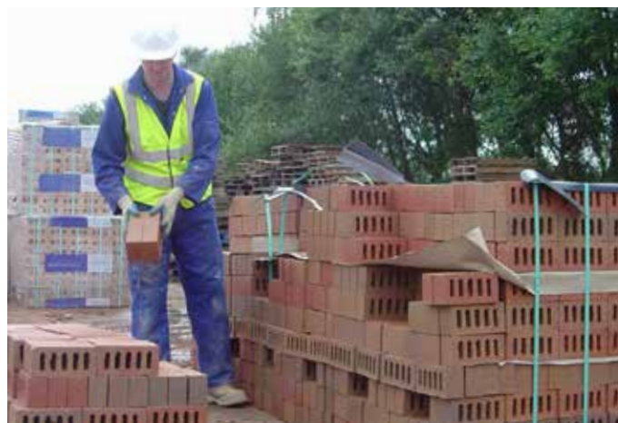
Correct blending from three packs or more concurrently as the work progresses.
