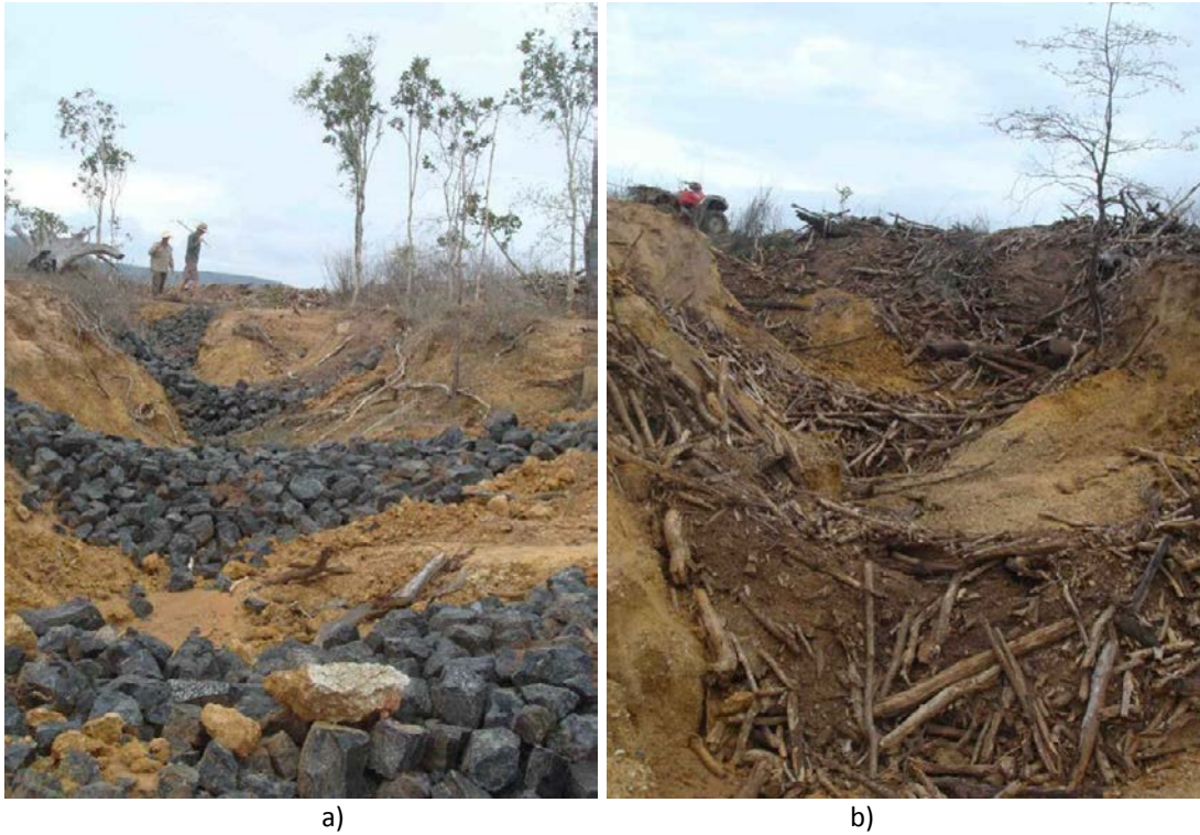
Figure 77 Examples of grade control structures used at a) CRGC1-34 utilizing sequential rock weir keyed into the bed and bank, and b) CRGC1-33 utilizing sequential small-wood weirs keyed into the bed and banks.
