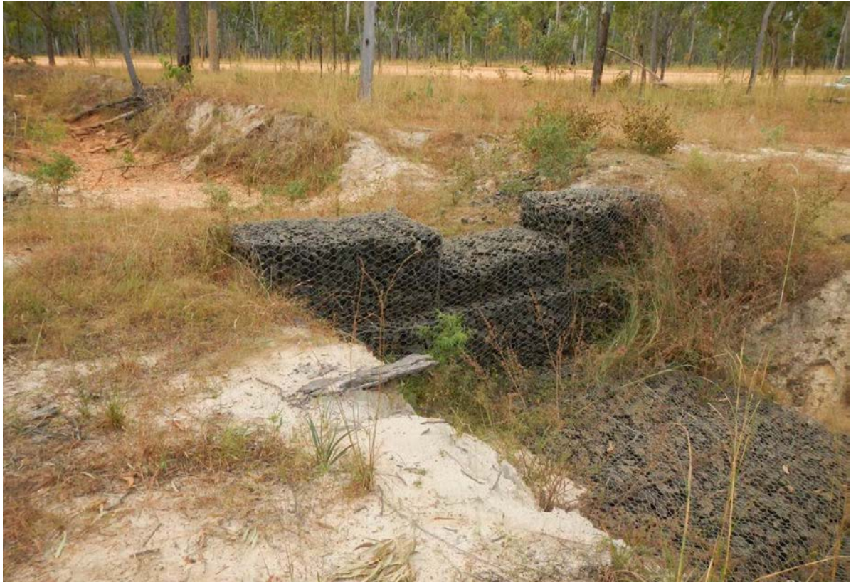
Figure 72 A rock gabion drop structure at a linear gully headcut below a road drain in the Normanby catchment. Note that the structure is not well embedded into the banks of the gully headcut.
