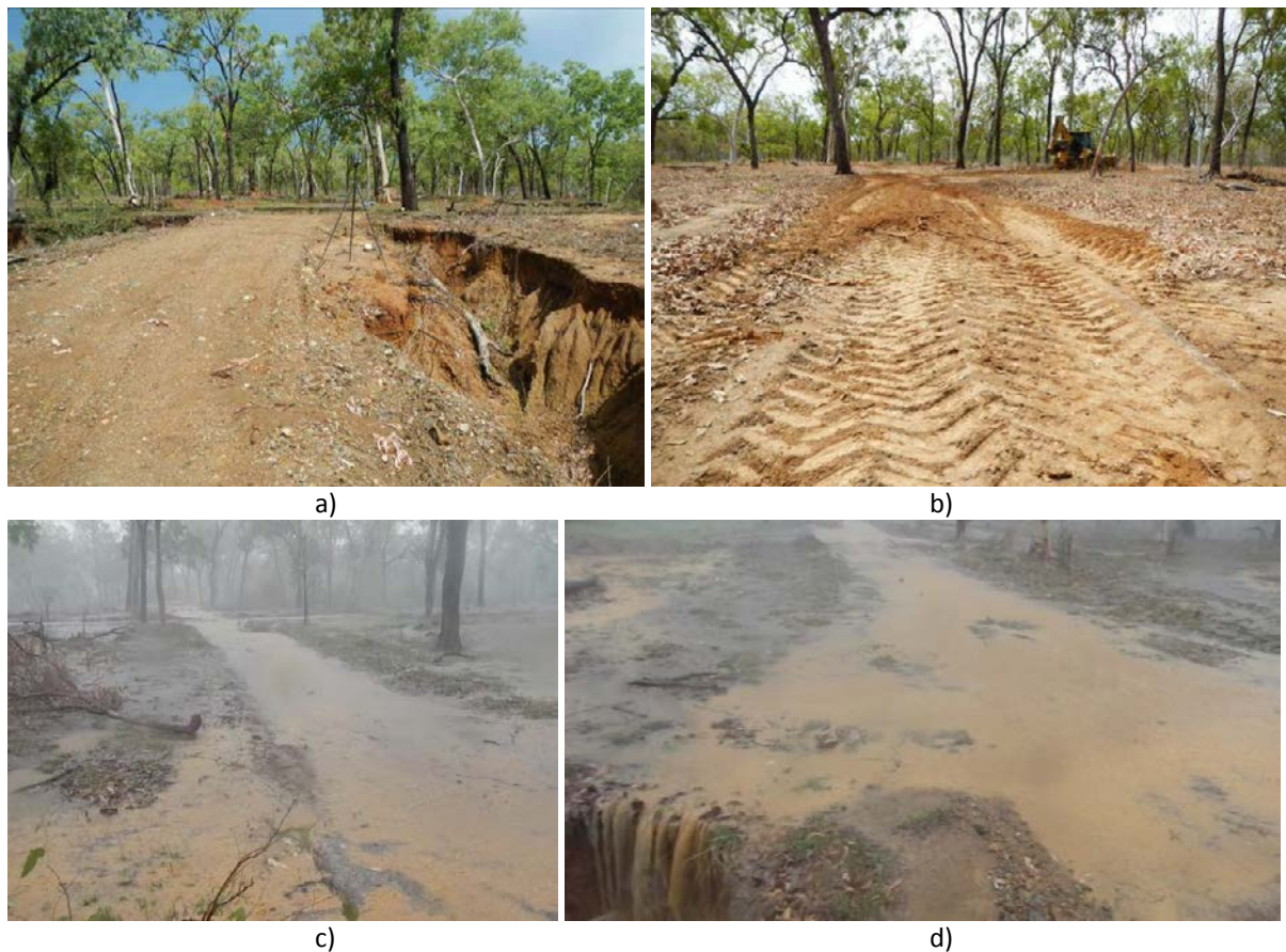
Figure 133 A major road choke point at RG30 where a) gully headcuts threaten the road from either side, b) water diversion banks (whoa boys) were installed to divert water off the road and away from the headcuts, looking downslope, c) water runoff down the road during a major rain storm filling the diversion banks and pits, looking downslope, and d) water runoff down the road bypassing and overtopping the diversion banks and continuing to feed the gully headcut.
