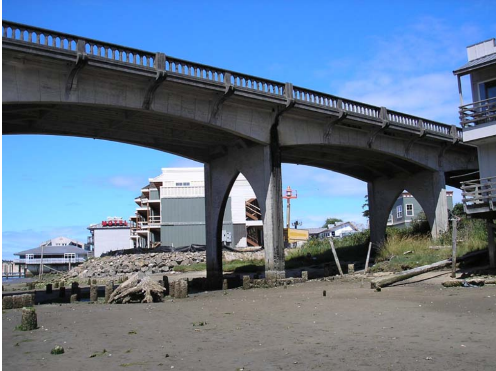
PHOTO 1: View of project site under bridge looking northwest. Condominiums west of the site are visible in background. Business east of the site is visible at right edge of photograph.
