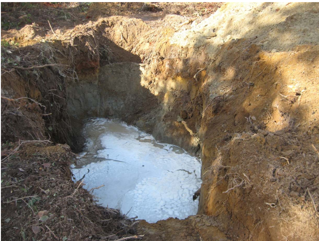
Photo 6. Typical water in test pits
