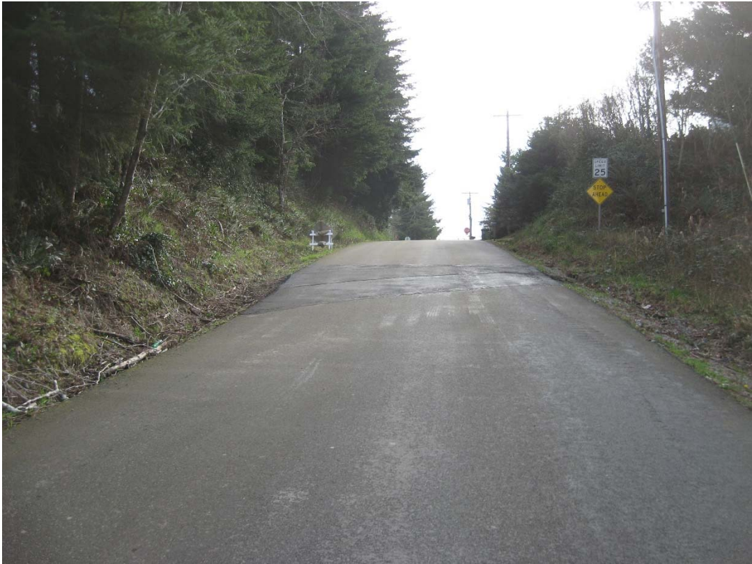
Photo 1. Offset on road pavement
