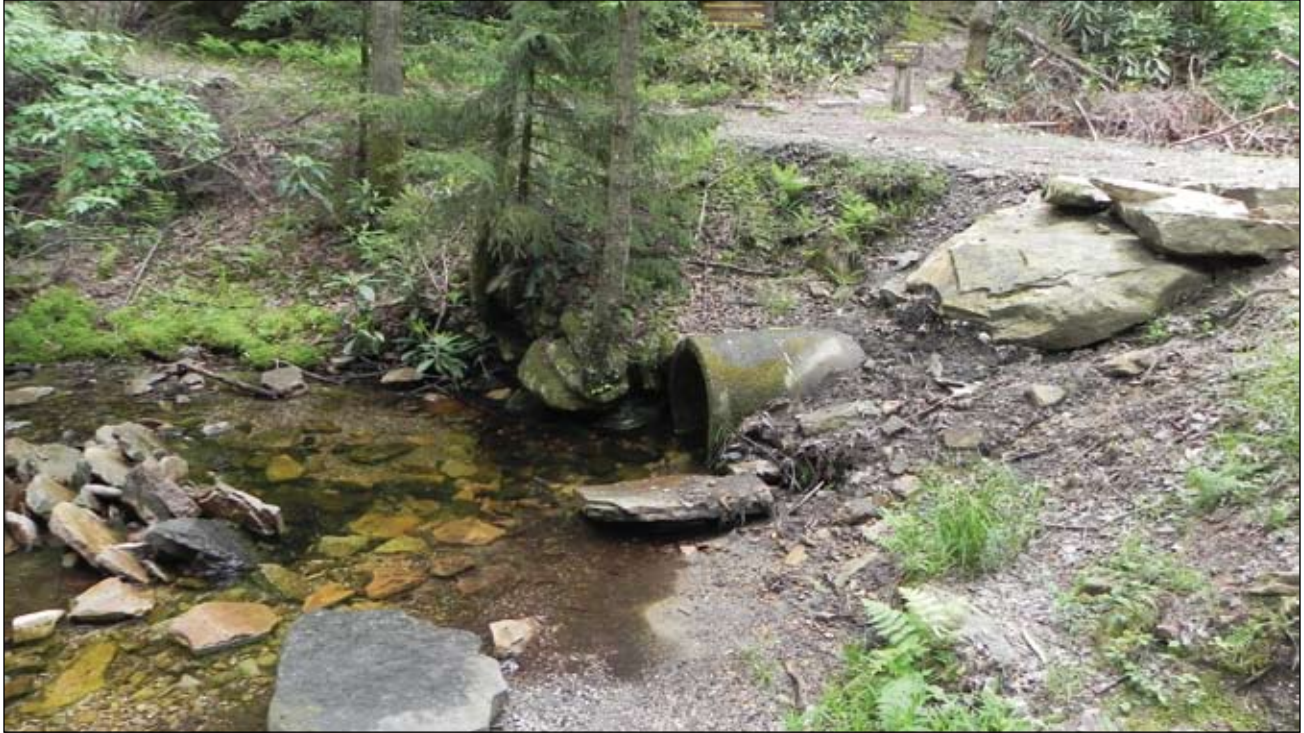
An old culvert. Land managers are beginning to replace culverts like this one with larger culverts designed to accommodate larger peak flows and allow the passage of aquatic organisms. Photo by Patricia Butler, NIACS and Michigan Tech, used with permission.
