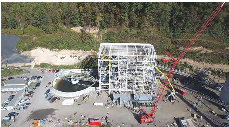
Ramaco Resources' Elk Creek prep plant is America's newest coal washing facility.
