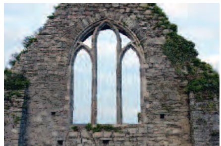
Decorated tracery window at the west gable of the Dominican Friary in Youghal.
