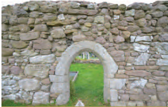
The 15th/16th century door inserted in the south wall of the nave with stone carved head above. The low pointed door with its finely dressed limestone surround stands out against the red sandstone of the earlier wall of the nave.
