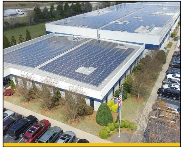
Hannah Solar Spartanburg Site.
