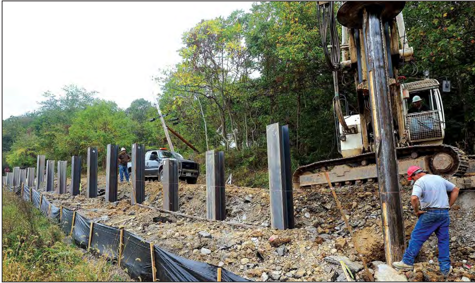
Workers from Alan Stone Inc. continue their drilling operation to set steel beams, on Monday, as part of the fix for River Road.
