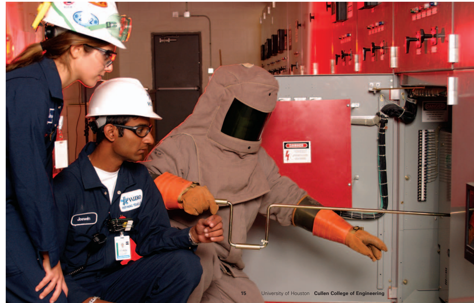
ISIP students Jeswin Manakalathil and Yassaman Ebrahimi rack a high voltage circuit breaker with D.C. “Frog” Smith (wearing an arc protection suit) in a substation at Valero.
