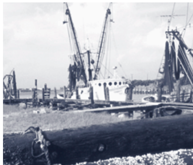
Shrimp boats viewed over old, barnacle-encrusted pilings at Conn Brown Harbor, Aransas Pass, Texas (Mr. William B. Folsom, NOAA, NMFS).
