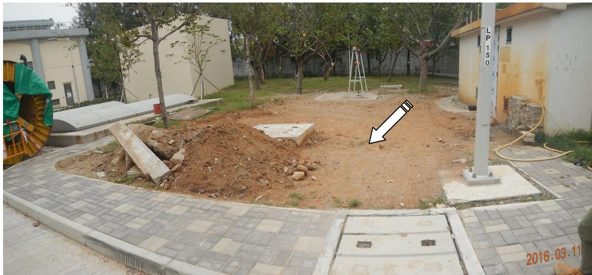
Photo no. G-09: Groundcover and Lawn were observed in poor condition during the site inspection.
