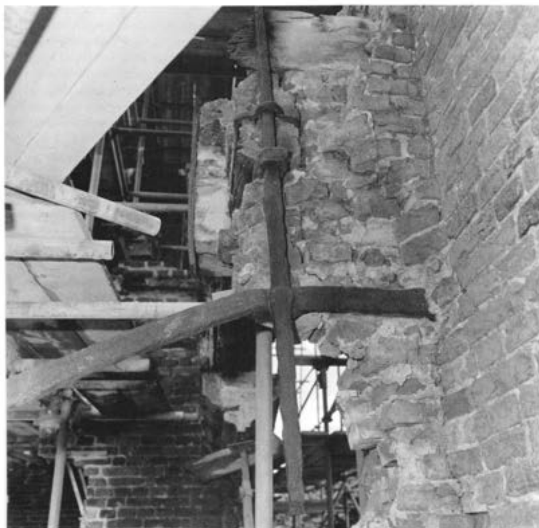
Plate 3 The east side of the east tower: a vertical iron rod runs through the fishtail plate on the soffit of an east-west timber which forms a lintel above the diaphragm arch at the back of the tower at first floor level. The rod is also stapled to the end of the timber, and runs up behind a north-south timber embedded in the east wall of the tower. Further restraint was provided by a strap riveted at a lower level to the rod and originally encased in the side of the tower (Nicolette Hallett).
