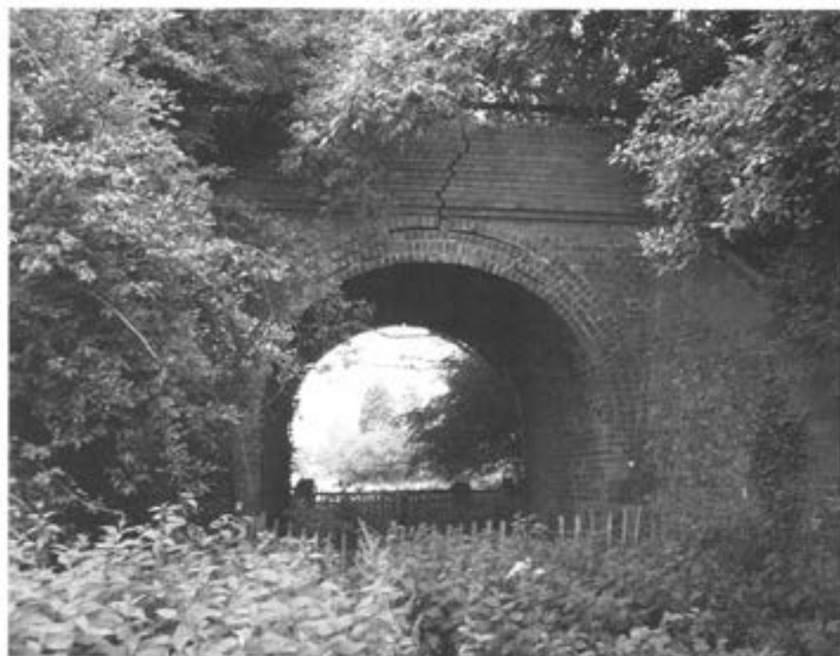
Plate 2. Underbridge no. 31/2076 on the Flich Way at Little Canfield suffering from major structural failure – EHER 40360. This bridge has now been rebuilt.
