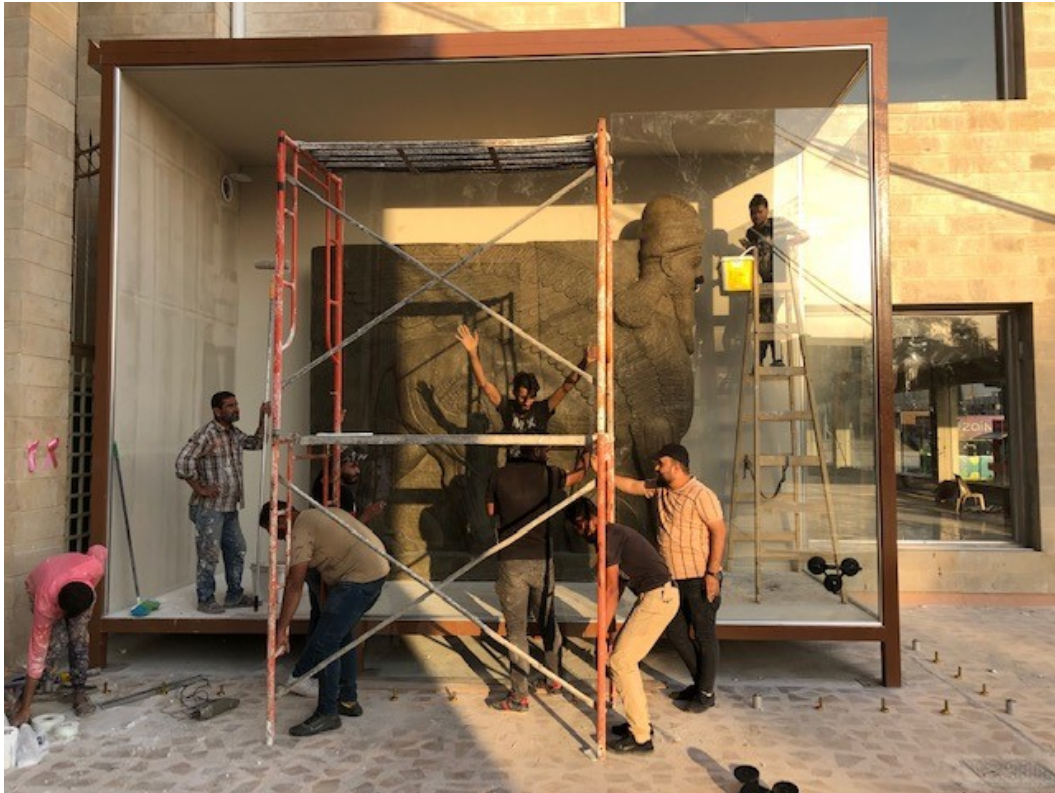
The installation of the lamassu at the entrance to the student centre © Adam Lowe for Factum Foundation
