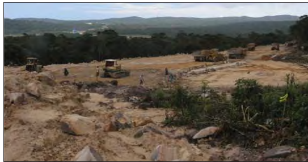
Fig. 3 Construction on the Bokor Plateau. 'Improvement' of a road to the Popokvil Waterfalls (© O. Kosterin).
