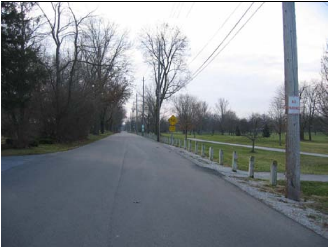
Figure IV.12 View looking south along Hartman Road, which defines the eastern edge of the Golf Course area. A considerable amount of the Foster Park street frontage includes the golf course edge along Hartman Road. For this reason, the character of the golf course landscape plays an important role in the overall identity of Foster Park. Also note the wood bollards that prevent parking on the open turf, signs and overhead utility lines. Courtesy Heritage Landscapes. (R- FWP-FOS_20061206_0196.jpg)
