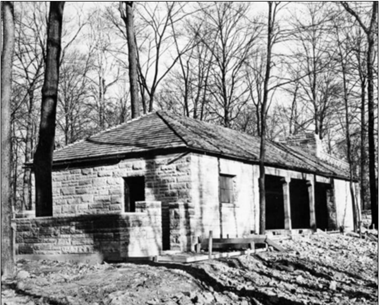
Figure II.15 View of the third pavilion under construction in Foster Park. Constructed in 1930, this pavilion was located in the southern portion of the park and set within a small woodland clearing to accommodate a growing demand for additional picnic facilities throughout Fort Wayne. Courtesy Allen County Public Library, Genealogy Division. (R- FWP-ALCA-Foster-Pavilion-ND.jpg)
