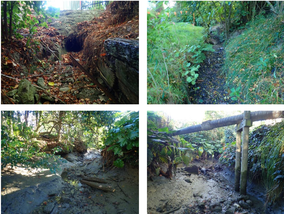
Figure 2-3: Photos of the upper and lower sections of intermittently flowing overland channel that receives the Seymour Rd/Turenne St overflows. The top left photo shows the combined stormwater-wastewater outfall.
