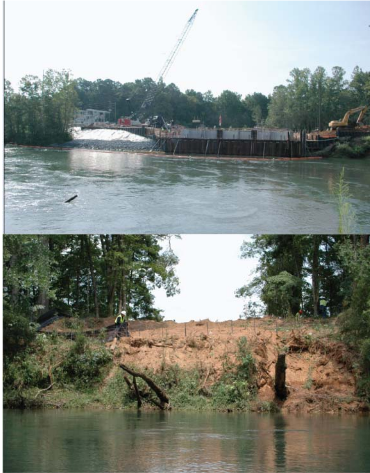
Plate 23. Construction of a new wastewater treatment plant (upper panel) at Holcomb Bridge on the Chattahoochee River, including a clear violation of sediment erosion control regulations (lower panel). Photo by E. Morris, 2008.
