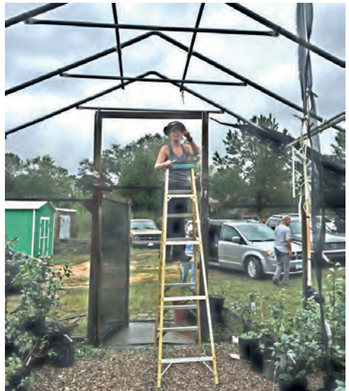
Christi Hankins cuts down old fabric ties in preparation for the installation of new shade house material. Though due for replacement, the cloth took a significant hit from Hurricane Sally.
